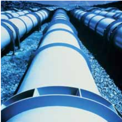
Monterrey City, Mexico Agua y Drenaje de Monterrey in Mexico is installing Danfoss VLT® drives in wastewater treatment plants, boost pump stations and water wells for both residential and commercial areas in Monterrey - the largest industrial city in Mexico with 3.5 million people. Benefits from VLT® operation of the pumps are energy savings of about 30% and also reduction of water leakage.
