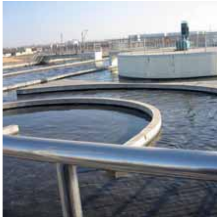
Xi'An No.3 Waste Water treatment, China Danfoss provided VLT® AQUA drives and MCD soft starters for Xi'An No.3 Wastewater treatment plant. It is one of three bundles of a retrofit project to improve the environment in Xi'An City of Shanxi province, China. The treatment capacity is 100,000 tons of sewage and 50,000 tons of recycled water per day.
