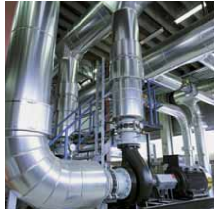
Izmir Geothermal District Heating System, Turkey VLT® drives operate the deep well and supply pumps in Izmir geothermal district heating. Applying VLT® drives leads to a very low electricity cost.
